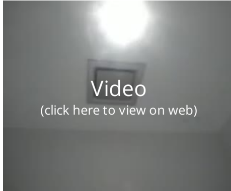
Exhaust Fan Condition: Operated normally at time of inspection
