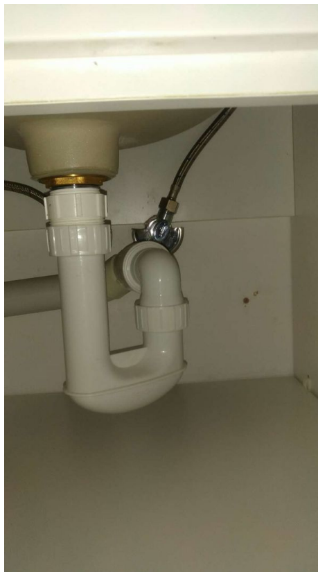
Sink Condition: Waste trap Appeared in serviceable condition at time of inspection
